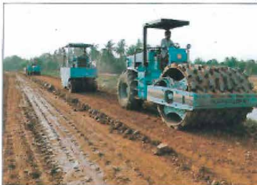
Cambodia: Compaction of the road surface. The road construction methods using Con-Aid in this area are the same as those used in South Africa and, as in South Africa, provide a high-quality, low-cost road by making use of in-situ materials, as well as materials normally considered unsuitable for road construction.
