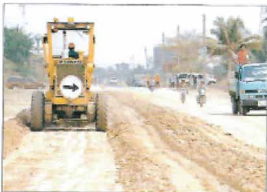
A Con-Aid road in the process of construction in a city in Thailand. Due to the high volume of traffic it is impossible to close the road and work has to be done without interfering with the flow of vehicles. The use of Con-Aid minimises this problem.
