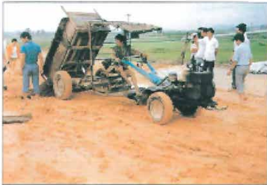
The making of a road in Mainland China with little or no mechanical equipment is shown in the photographs above.
